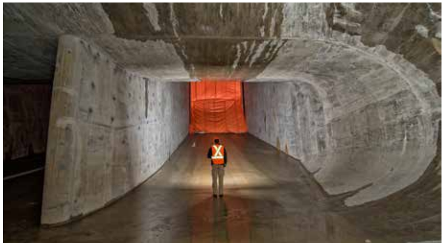
An OPG employee examines the concrete draft tubes of Smoky Falls Generating Station.
