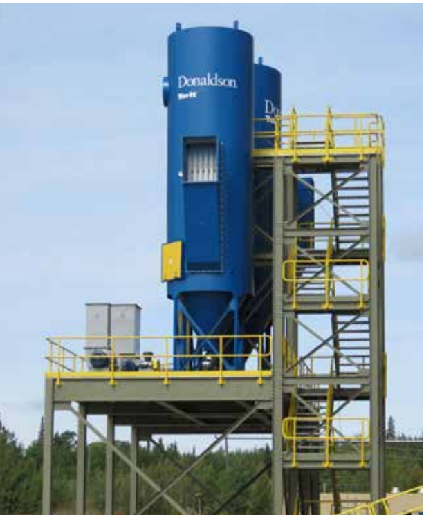
Dust collectors at Atikokan Generating Station
