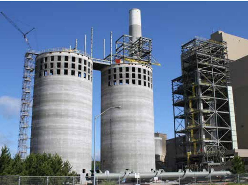
Biomass storage silos at Atikokan Generating Station.
