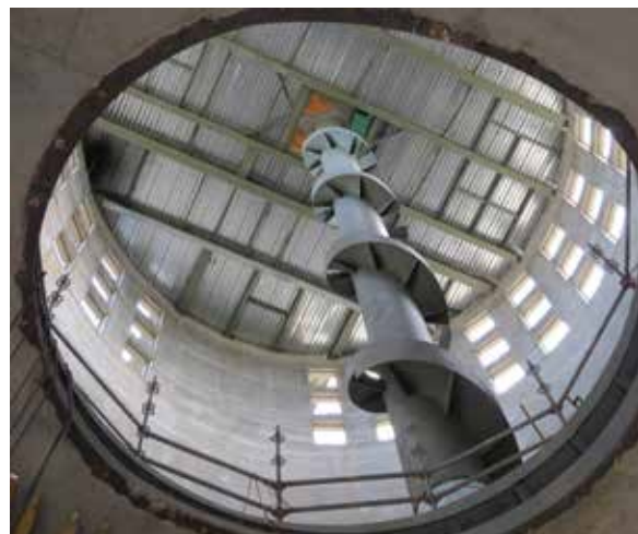
Inside view of wood pellet silo at Atikokan Generating Station
